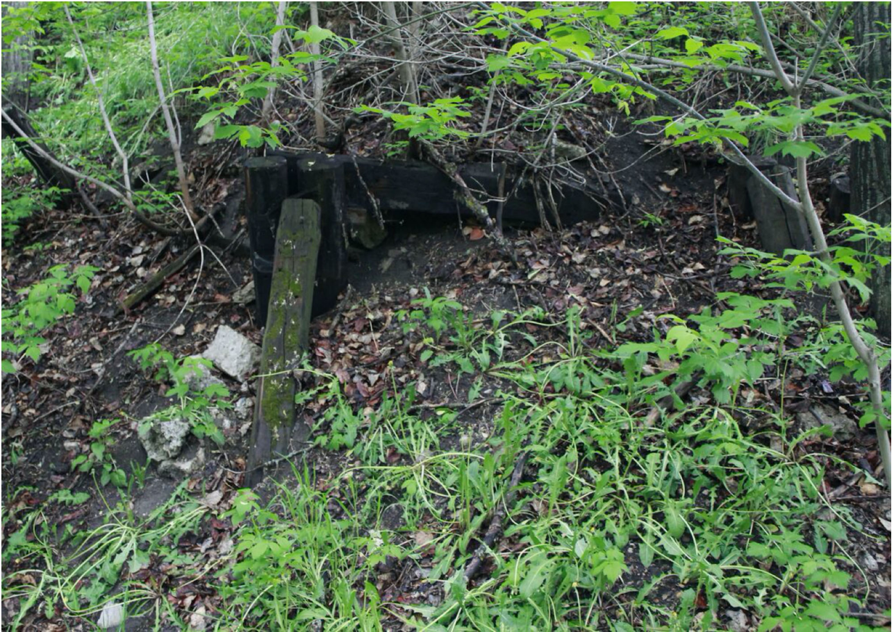
Figure 6.1. The decaying and growing entrance to Twin City Coal Mine (photo by Haeden Stewart). [This figure appears in color in the online issue]
